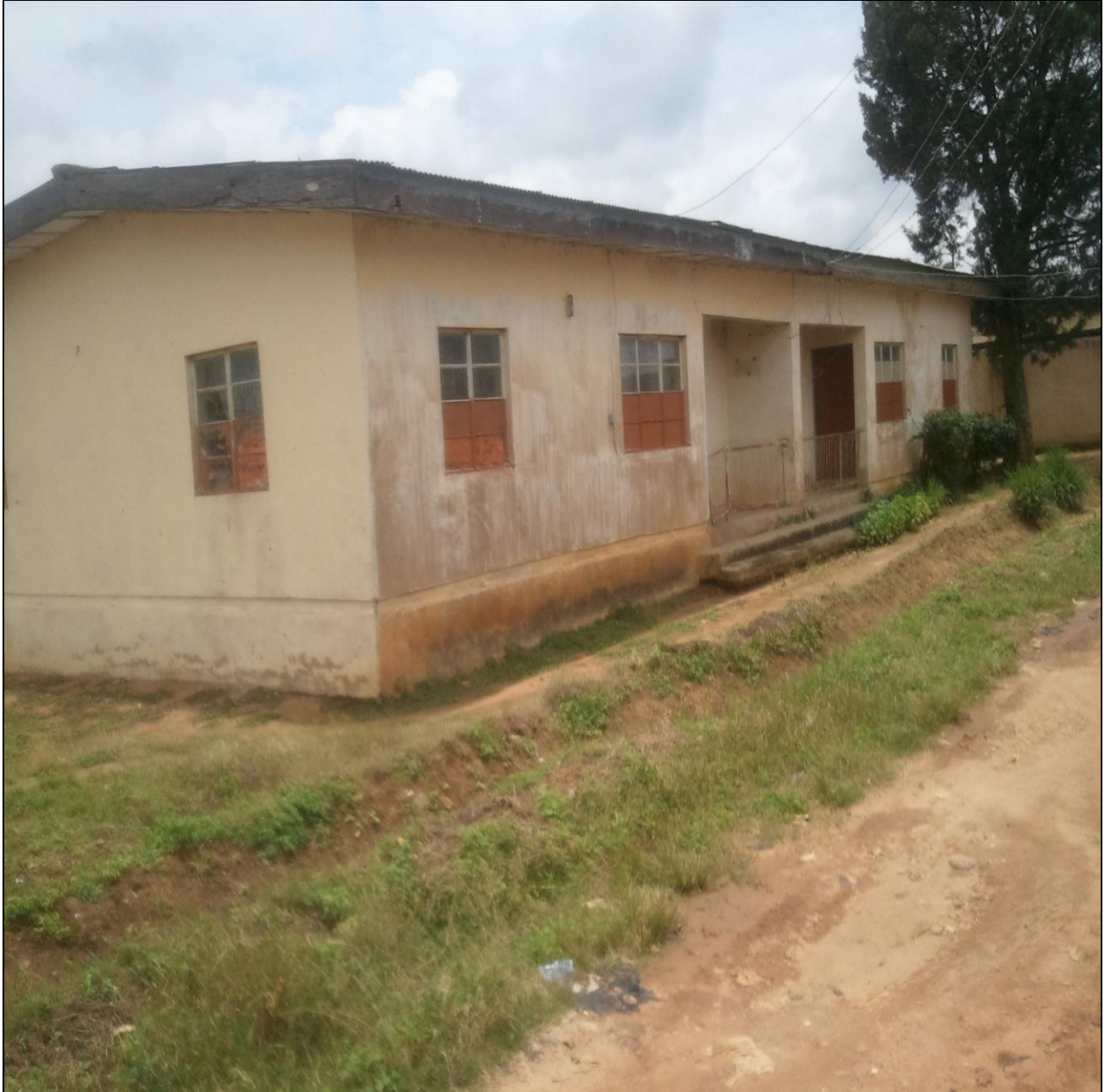
Plate 2: Typical existing Block of Semi-Detached House at Miango State Low Cost without Alteration or Renovation Source: Field Survey 2014.
