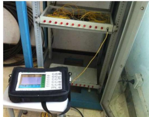
Fig. 3. OTDR connected to fiber under test
