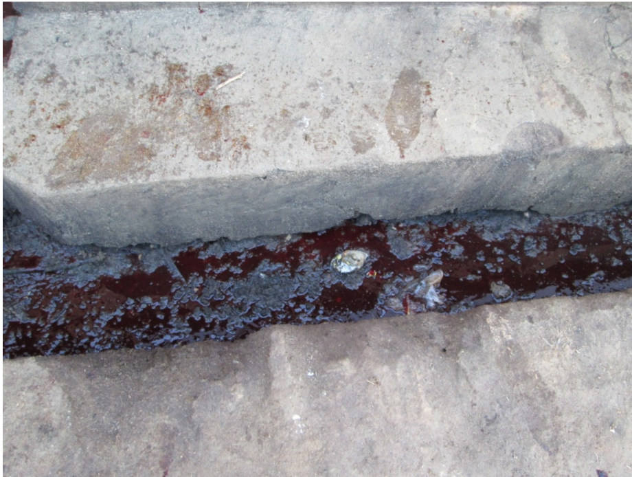
Plate 3. Slow moving effluent in one of the drainages at the Abattoir
