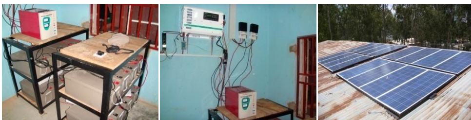
Figure 33: Batteries, Inverter and Solar Panels-Courtesy TfT Team
